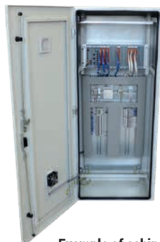
Example of cabinet for smaller substation
